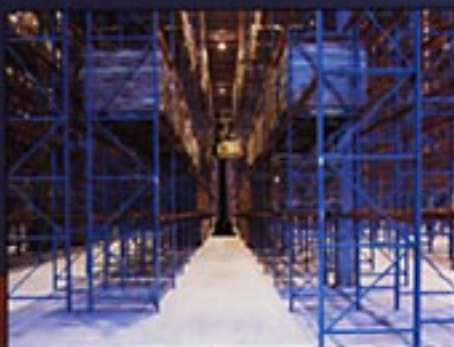
Hybrid System installation at Quality King Company, Long Island, New York.
